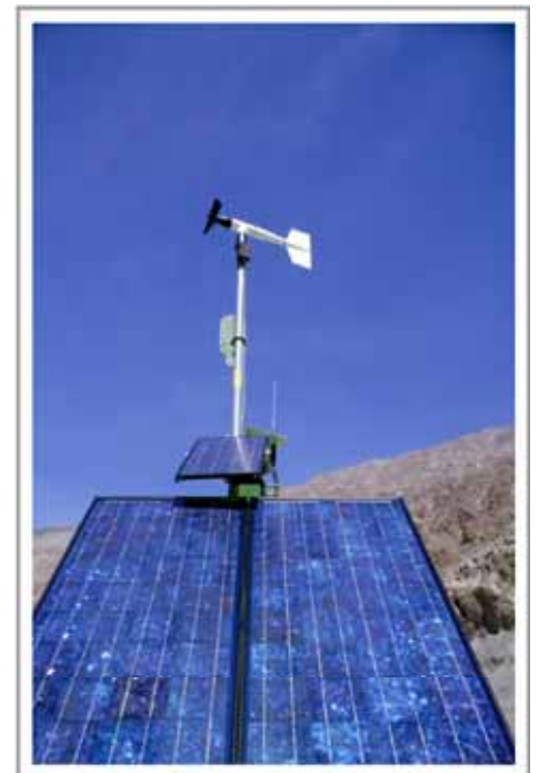
Photovoltaic solar panels
